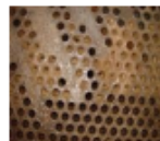
A badly scaled/fouled heat exchanger
